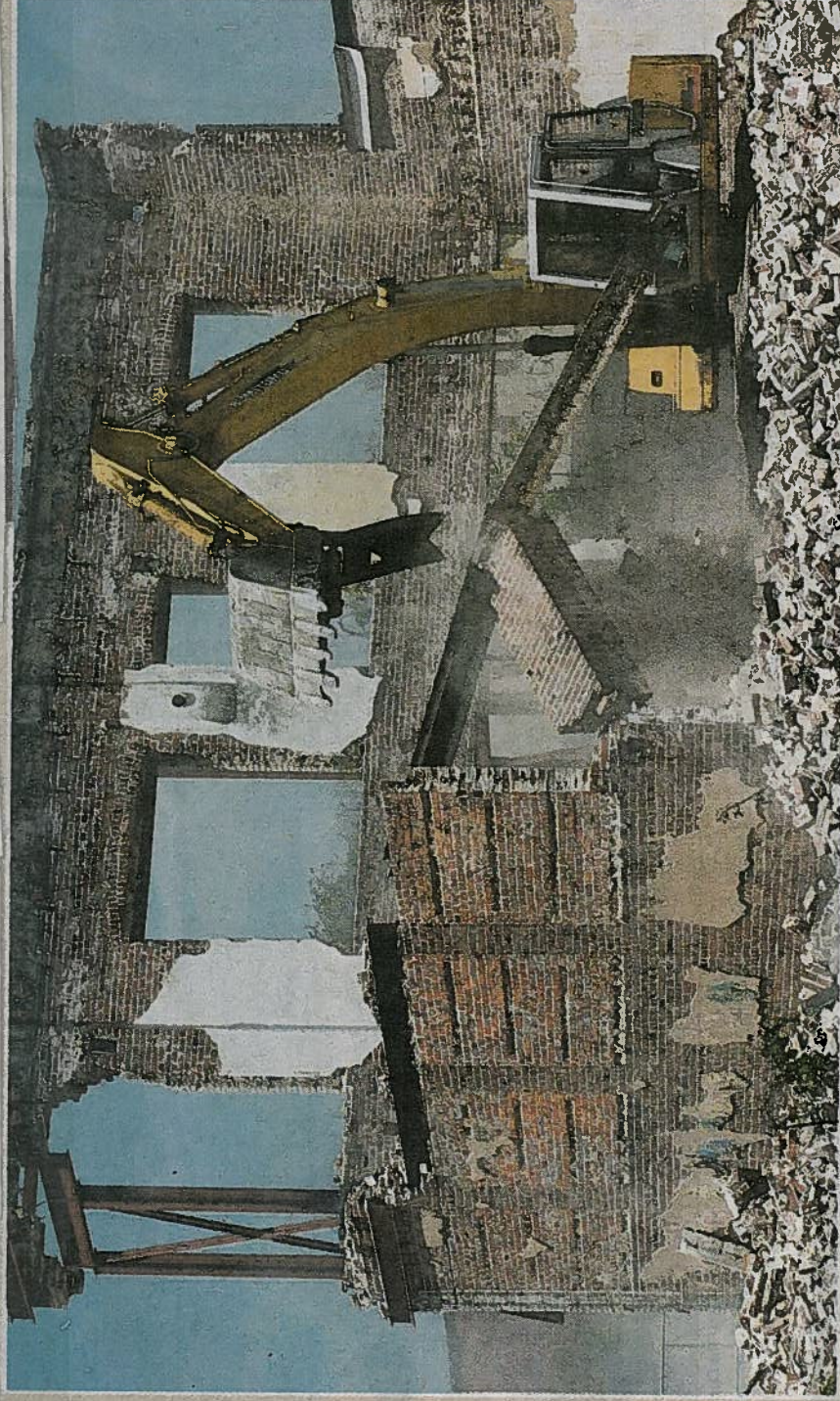
Eddie Taylor of Donaldson Construction Inc. of Jackson uses a backhoe on Wednesday to tear down a building at 230 Farish St. near downtown Jackson. The demolition is part of the Farish Street Entertainment District project.
